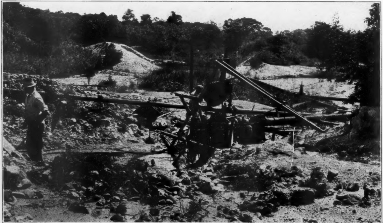
Upper Left Shows Receiving Tank and Settling Tank. Lower Shows Sump Pit Guarded by Iron Bars to Keep Out Large Stones
